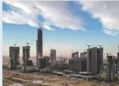
Central Business District of the New Administrative Capital, Egypt OVM supplied PT system.
