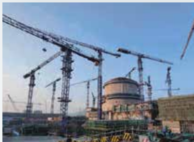
Taiping Nuclear Power Plant, China OVM supplied nuclear PT system, aircraft-impact-resistant rebar coupler, and specialized construction.
