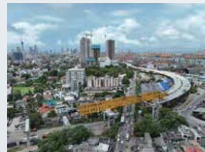
Port Access Elevated Highway Project, Sri Lanka OVM supplied PT system, HDPE pipe, bearings, equipment, expansion joints and technical support.
